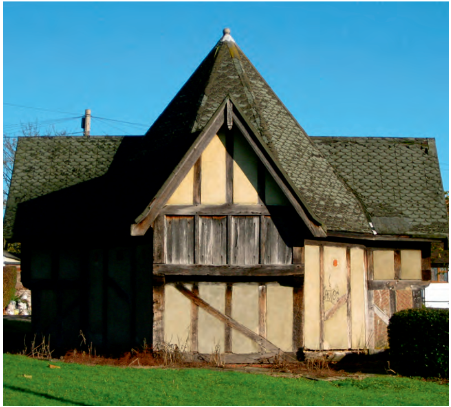
Many of the well house's timbers are badly decayed and fallen away
