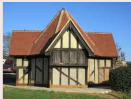
The restoration work proved more costly than originally estimated because of the extent of rotten timbers and crumbling brickwork
