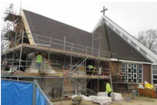
Work in progress: Construction nearly complete on a 100-seat extension to Barnet's Roman Catholic Church
